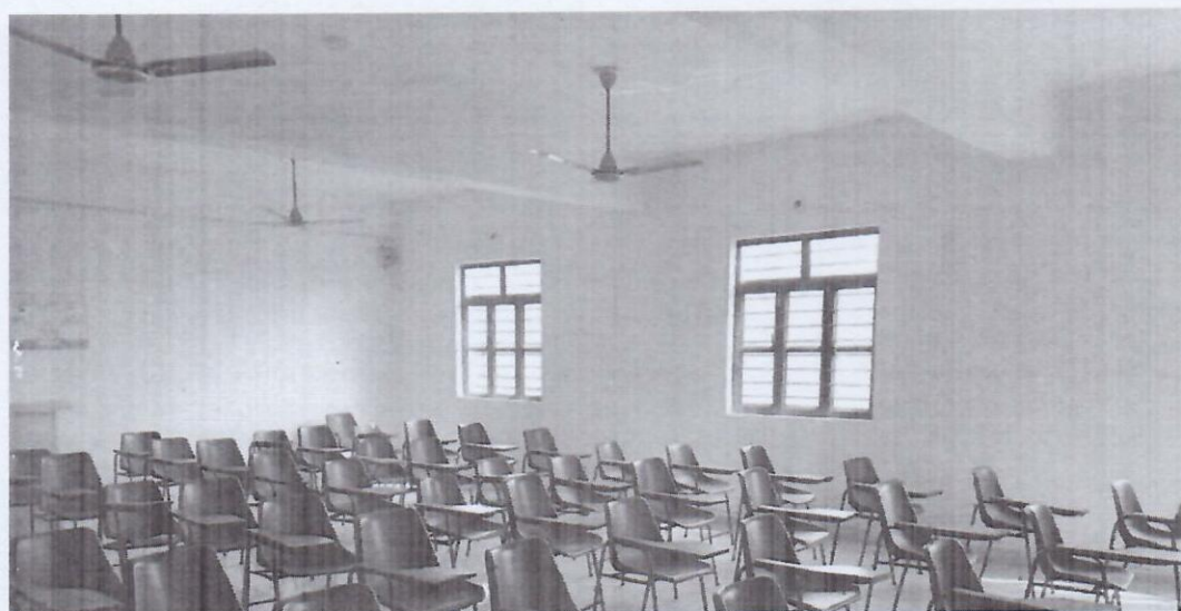
Old Type Ceiling fans are installed in the classroom
